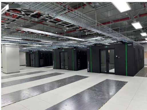
Main server room
