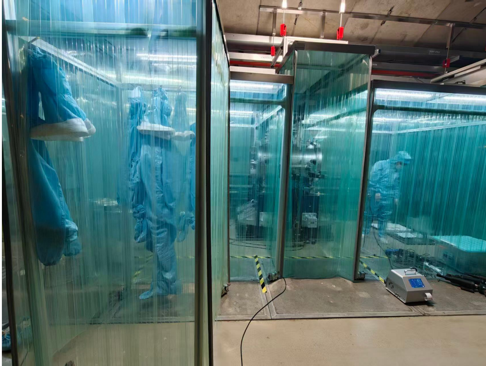
Local clean room for M1 installation
