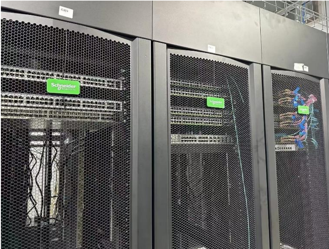
Access Switches @ DAQ server room
