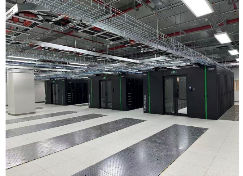
Main server room at shaft 5
