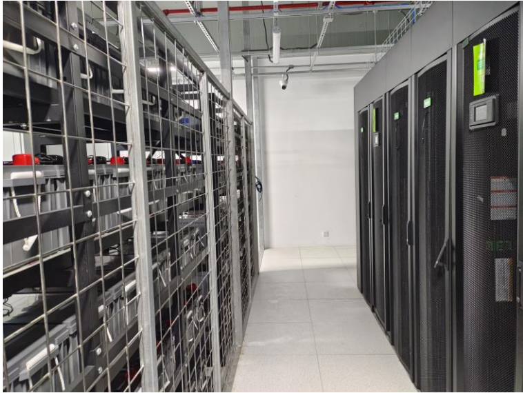
DAQ server room at shaft 4
