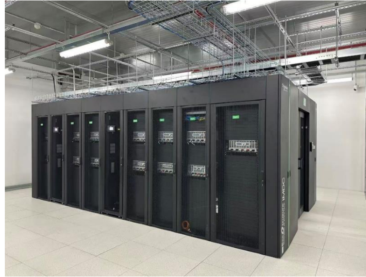
DAQ server room at shaft 5
