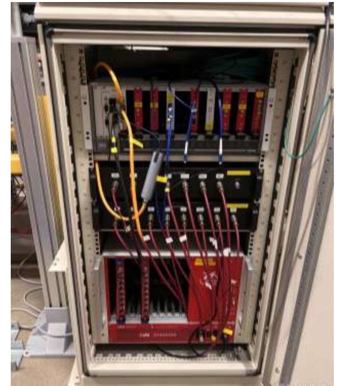
Data Acquisition and Control Cabinet
